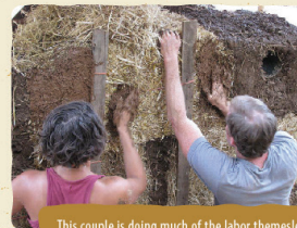
This couple is doing much of the labor themselves, saving them lots of money on construction costs.
